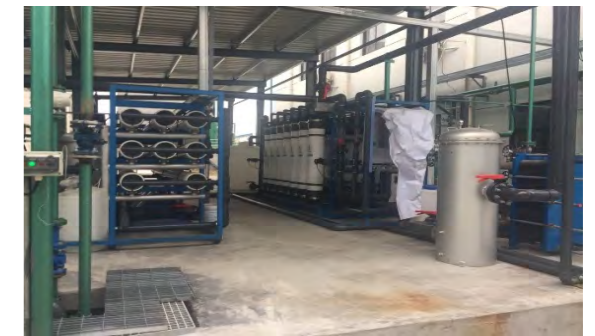
After improvement: after treatment, the wastewater enters the advanced treatment system and is reused in the cooling water circulation system.
