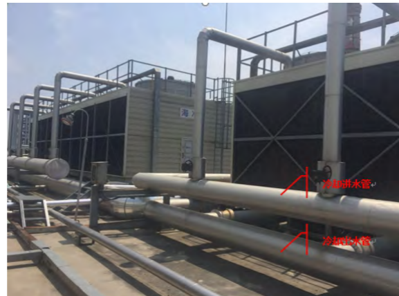
Circulating Cooling System of Centralized Cooling Tower
