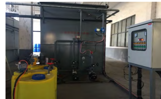
Before improvement: the reclaimed water reuse project had not been implemented, and the wastewater was directly discharged into the pipe after being treated by the sewage station.
